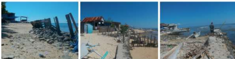
Figure 7. Some evidences of shoreline change by abrasion and accretion at Barrangcaddi at 2018. The ruin of shore protection structure (left), the houses become near to shoreline (middle) and right, the second layer of concrete build to protect the shore but damage by erosion (Photos by author)
